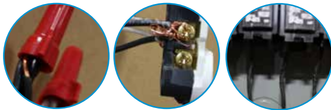
Improper solid wire connection.
