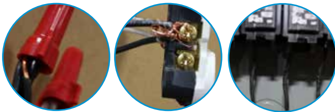
Improper solid wire connection.
